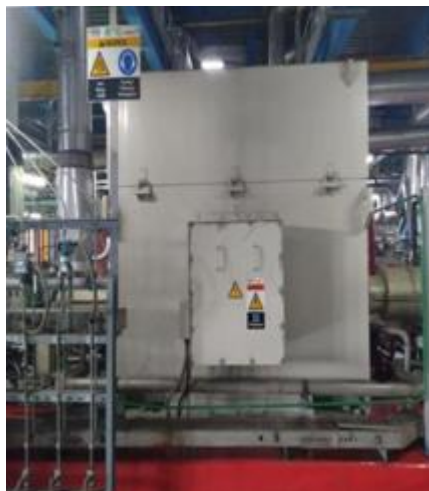
Gambar 2. Motor Pompa Boiler feed pump
