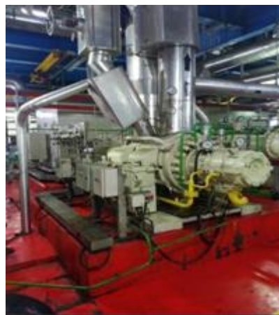
Gambar 4. Mesin Boiler Feed Pump
